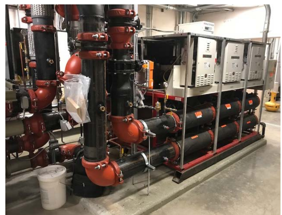
Figure 2: Three remaining Multi-stack chillers
