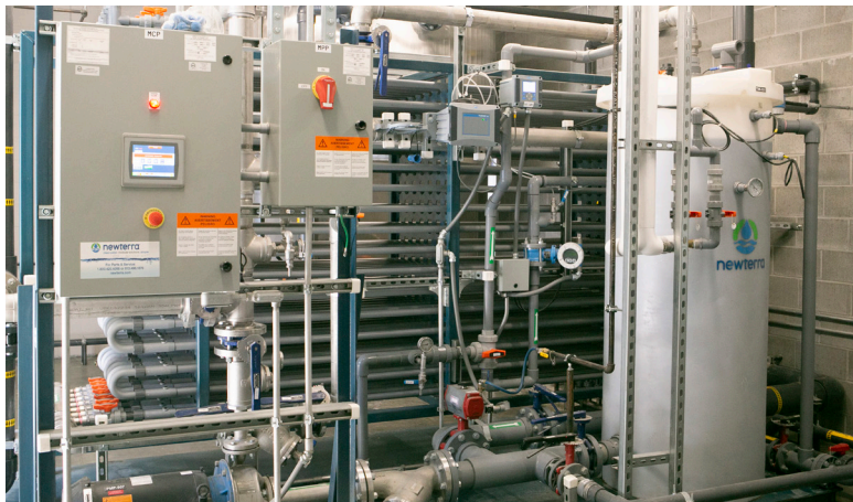
Wastewater Treatment Facility – Victoria
