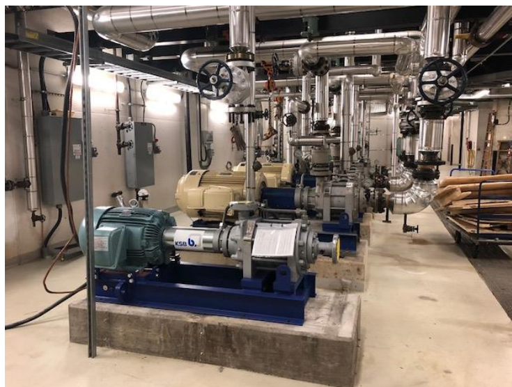
Photo of the new feed water pump, enabling a reduction of 241,000 kWh's of electrical savings each year.
