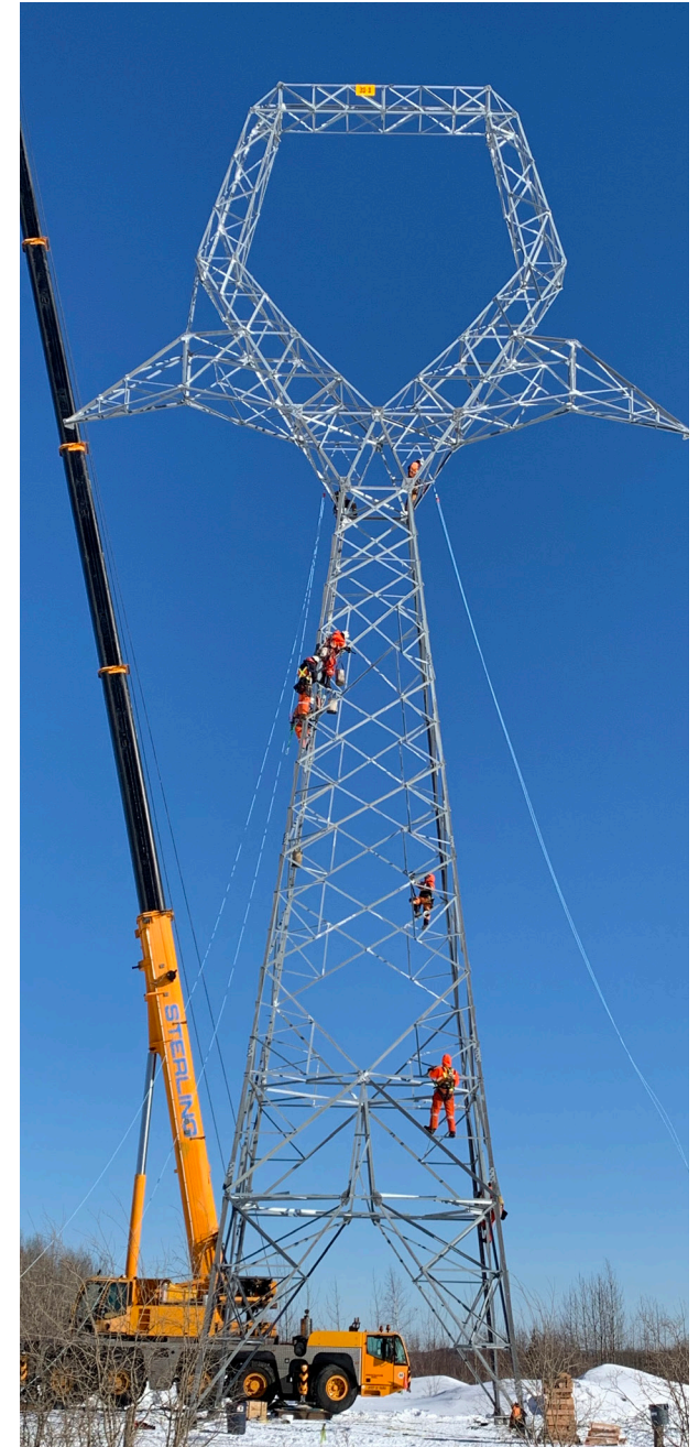
Upgraded Transmission Lines withstand icestorms
