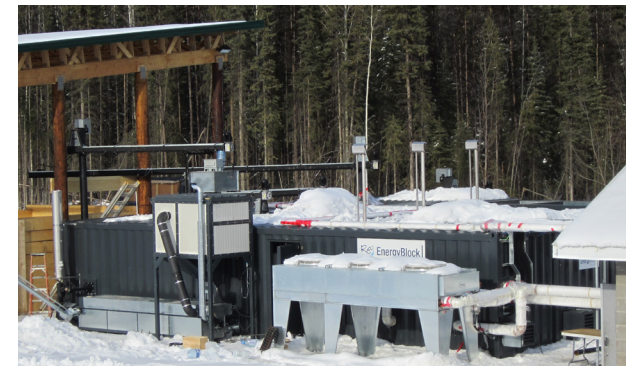
Biomass Plant at Kwadacha
