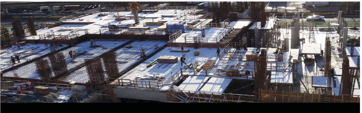
Crews working on the new mental health building at Royal Columbian Hospital.
