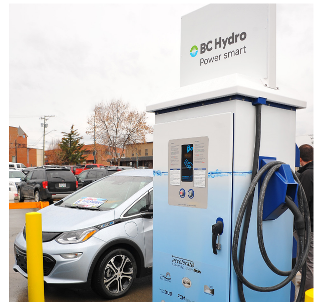
DC Fast Charge Station.
