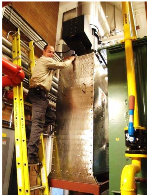
RJH Assistant Chief Engineer, Sacha Menard, inspecting the Royal Jubilee Hospital Flue Gas Condensing Economizer
