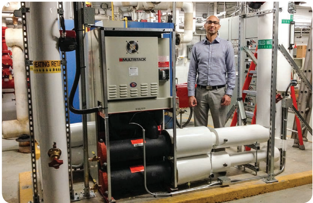
Sunny Brar, our FortisBC-funded Energy Specialist, helped build the case and access funding for our new dedicated heat recovery chiller at Head Office.
