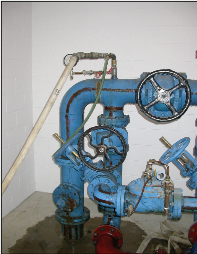
Plate 2. The raw water tap within the Fort St. James pump house.
