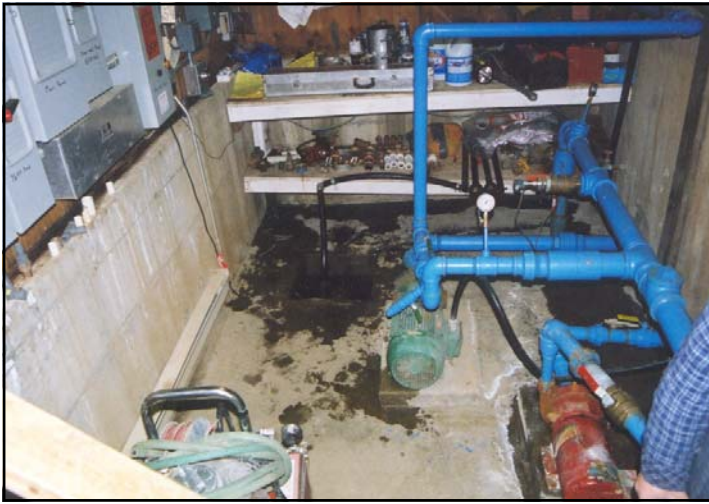
Plate 2. A picture of the raw water tap inside the Buckhorn pump house.
