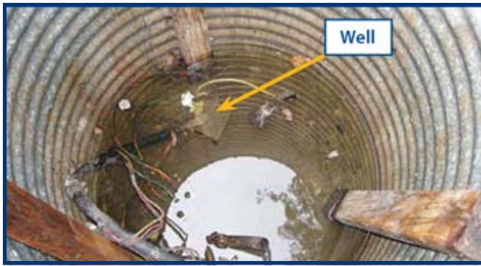
Figure 3. Water and debris in well pit
