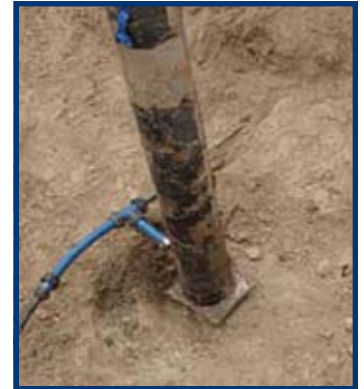
Figure 6. Pitless adapter works installed below frost line
