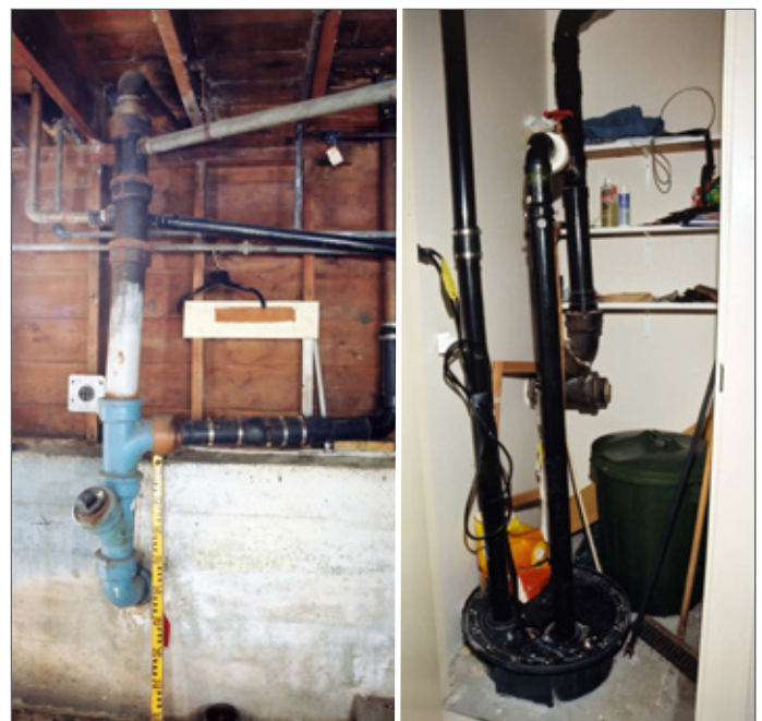
FIGURE 3 Sewer outlet pipe (Left) FIGURE 4 Sewage lift pump (Right)
