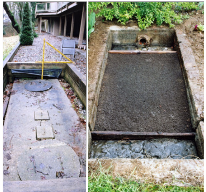
FIGURE 6 Newer style septic tank (Left) FIGURE 7 Old style septic tank lids removed (Right)
