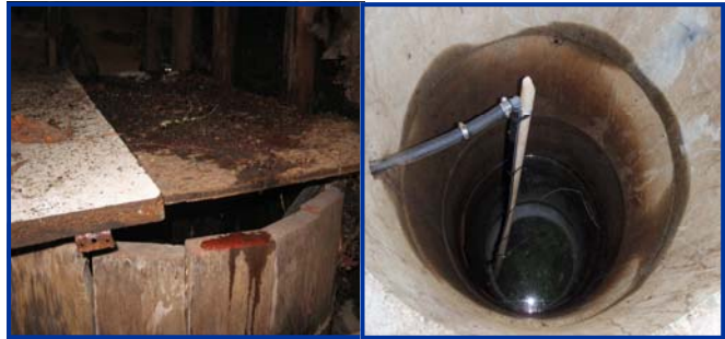
Figure 8: Water able to seep into well through the casing
