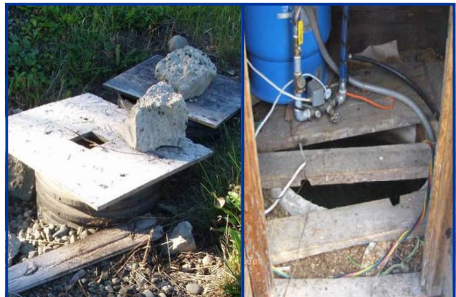
Figure 5: Improperly covered wells
