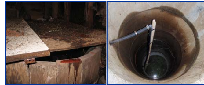
Figure 8: Water able to seep into well through the casing
