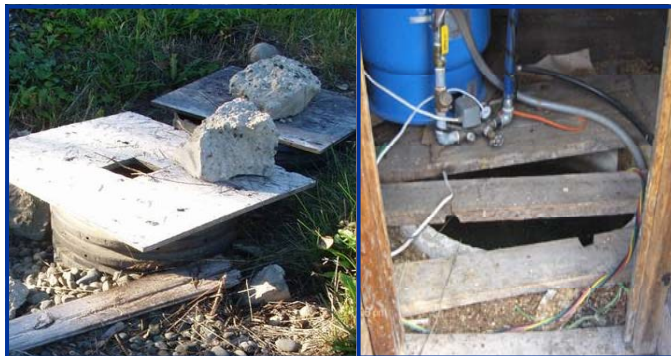
Figure 5: Improperly covered wells
