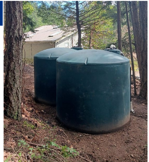
Figure 1 Cisterns storing rainwater collected off a roof. Credit: Leia Fougere (WLRs).
