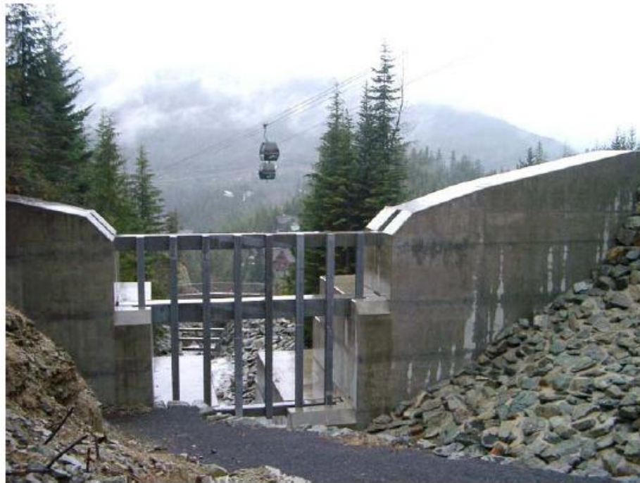
A debris barrier on Whistler Creek, Whistler, B.C., designed to retain 30000 m 3 of debris.
