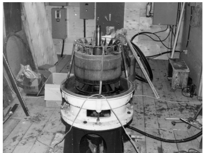
Pump disassembled for maintenance.
