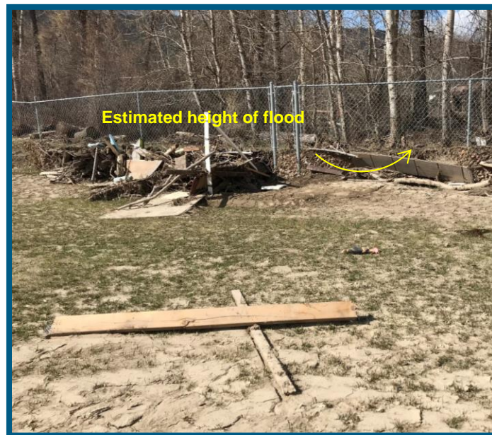
Photograph 3: Example of sediment and flood debris. Material deposited against chain link fence surrounding a sports field. Note the estimated height of the flood water mark.
