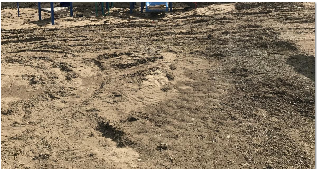
Photograph 8: Significant soil deposition in playground and surrounding area of Central Elementary School, looking east.
