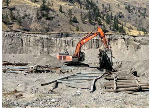
NR-73 bridge removal, initially thought to be bridge railing but was bridge with deck
