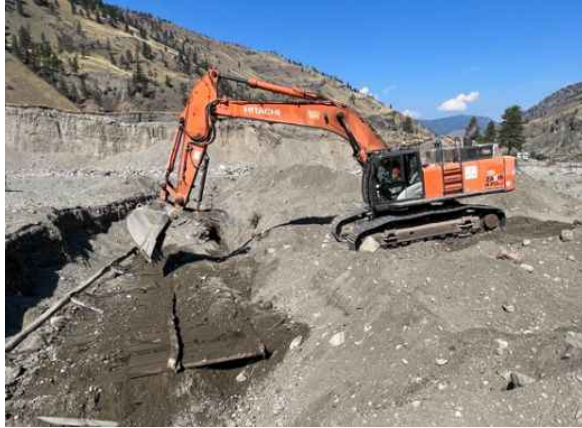
NR-73 bridge removal, initially thought to be bridge railing but was bridge with deck
