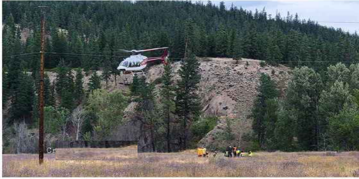
Linear debris removal
