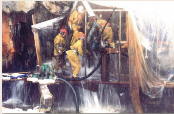
Photo 5: Drillhole experiencing artesian flow conditions.
