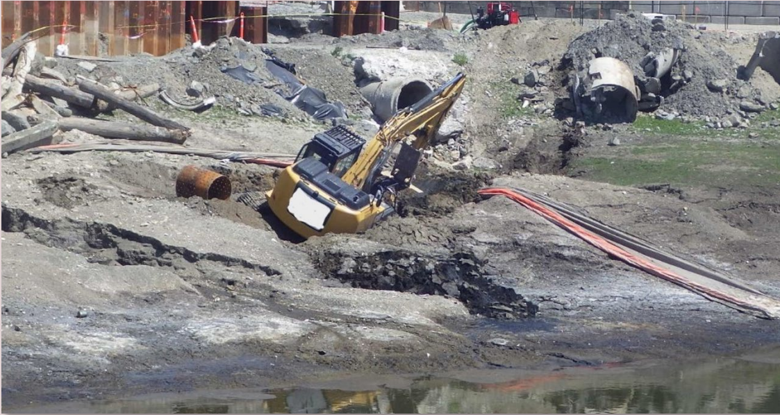
Photo 10: Excavator stuck in upstream slope, causing an undrained slope failure.
