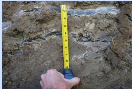
Photo 8: Example of hydraulic fracturing at Barker Dam.
