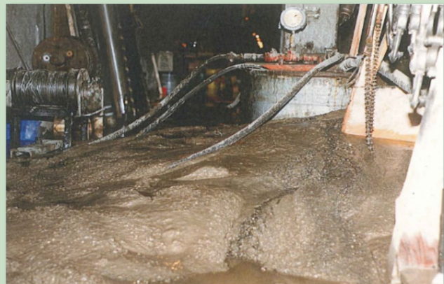
Photo 6: Core materials washed out of borehole.
