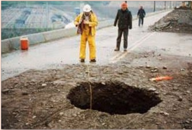
Photo 9: Sinkhole at WAC Bennett Dam. Prompt action prevented a dam breach. Photo by Ray Stewart.
