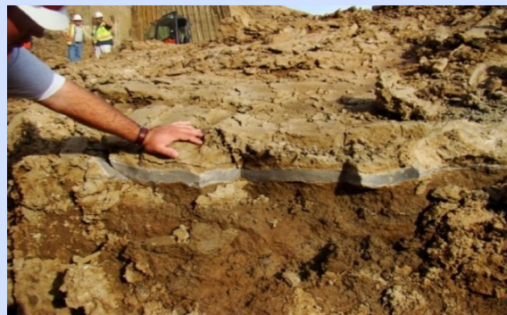
Photo 7: Example of hydraulic fracturing at Kentucky Dam.
