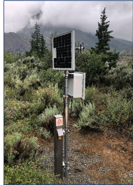
Photo 1: Solar-powered piezometer used to monitor water pressure inside a dam embankment.
