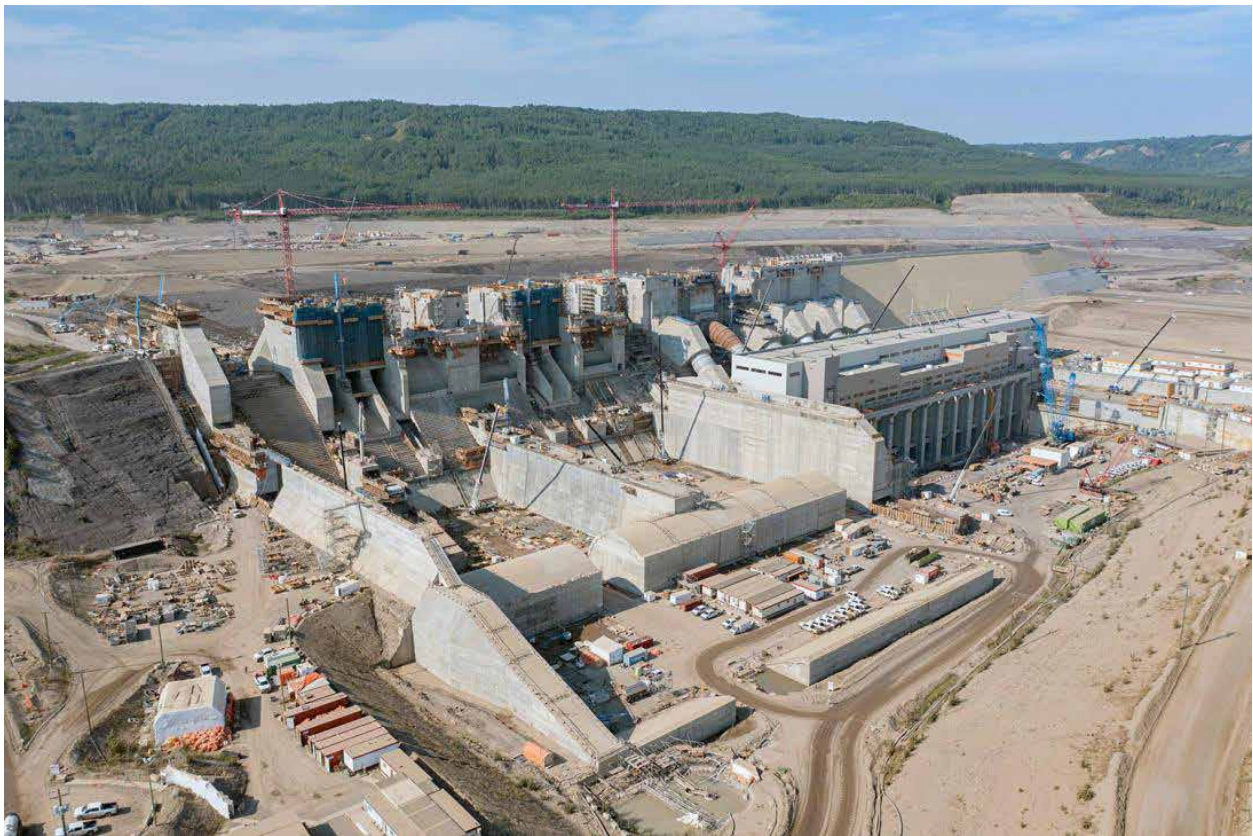
Photo 7 – Site C – View of the spillway, penstocks, powerhouse and operation building (Photo credit: 2017 Site C Clean Energy Project)
