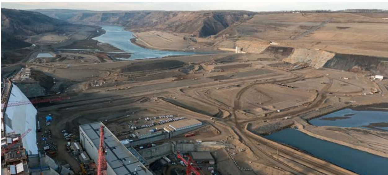
Photo 6 – Site C – view of Main Earthfill Dam and Cofferdams, Powerhouse and RCC Buttress. (Photo: BC Hydro)
