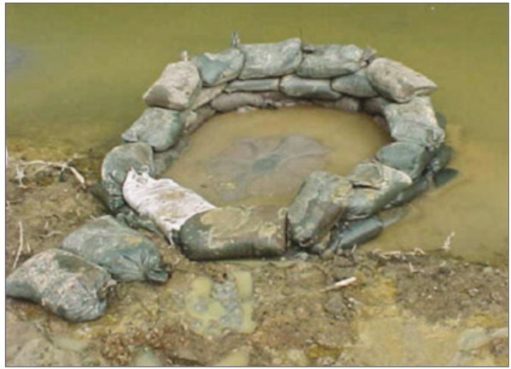
Sandbags Surrounding a Boil on Downstream
