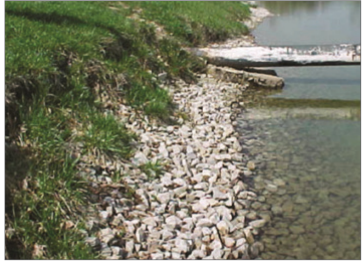
Wave Erosion on an Unprotected Face of a Dam
