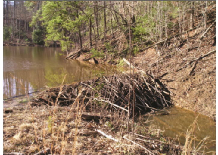
Blocked Spillway Channel of a Dam
