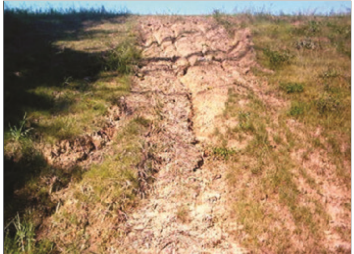
Erosion on the Downstream Face of the Dam
