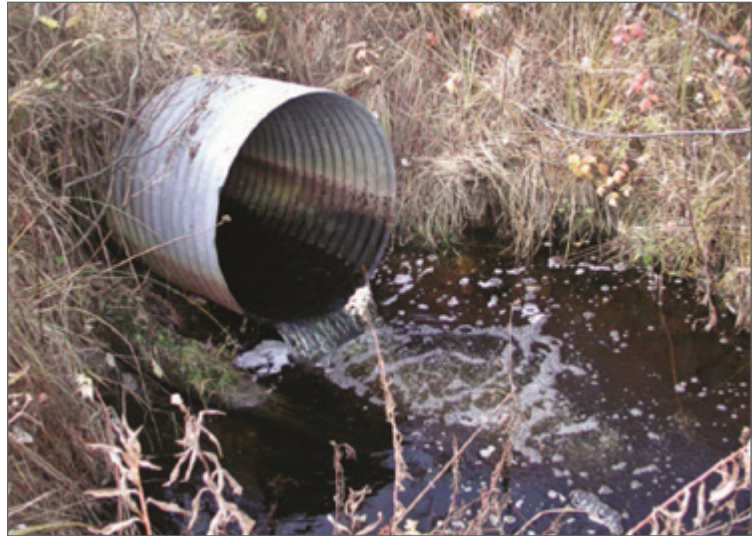
A Scour Hole at an Outlet Erodes Toe of Slope.
