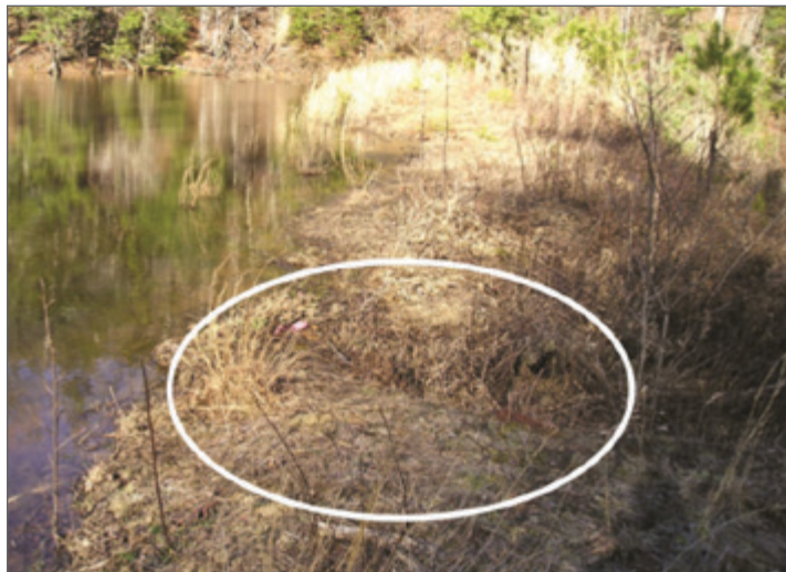
Low Areas in Crest Will Reduce Freeboard
