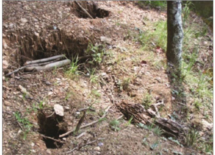
Rodent Holes on the Face of the Dam
