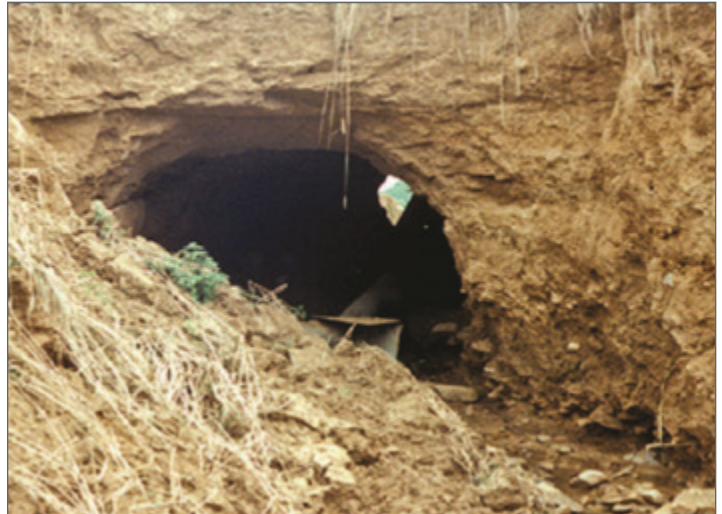
Piping of Water Alongside an Outlet Pipe
