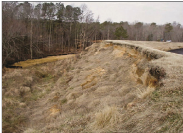
Slumping on the Downstream Face
