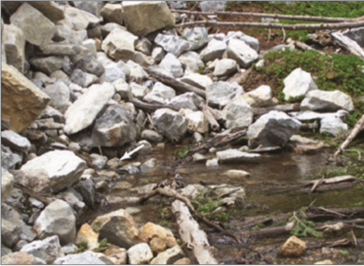
Water Piping Through Toe of Embankment
