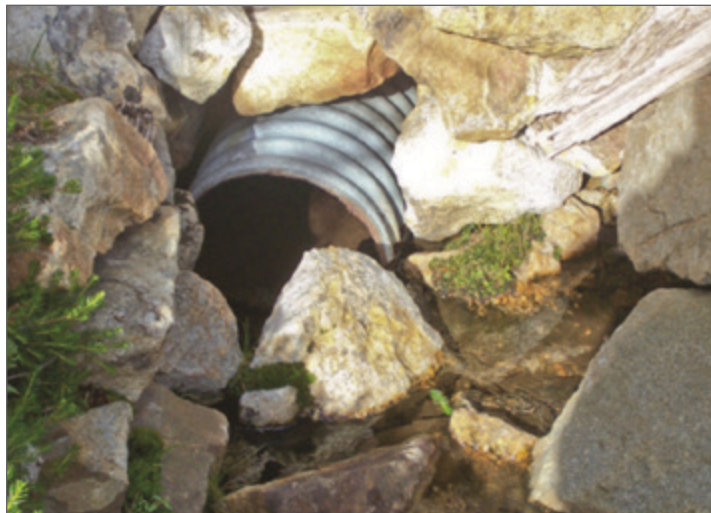
Rock Failure Around an Outlet Pipe
