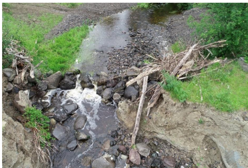
Photo 2: Valley Pond (Upper) Dam breach
