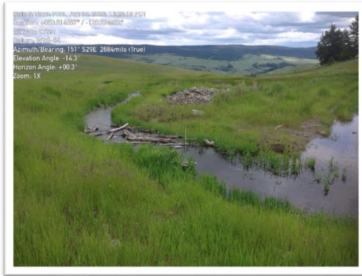
Photo 5: Debris in the spillway and high-water level at the Ussher Creek Dam (looking southeast)
