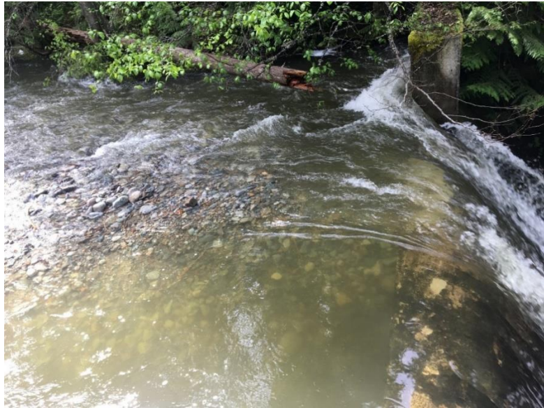
Photo 12: The sediment load has reached the spillway sill of the Rover Creek Dam
