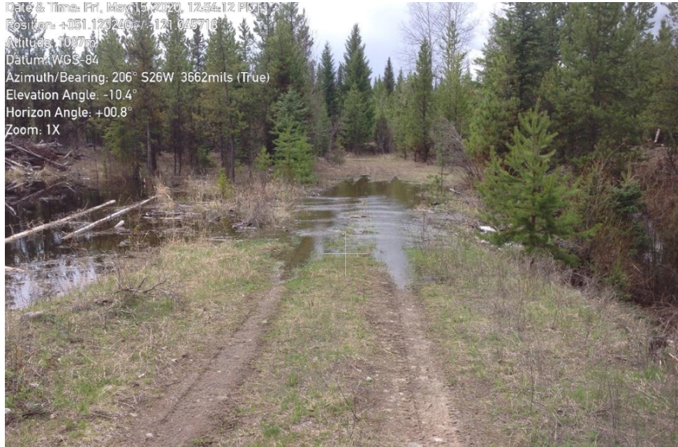
Photo 4: Overtopping of Goldie Lake Dam (looking south south-west from right bank)
