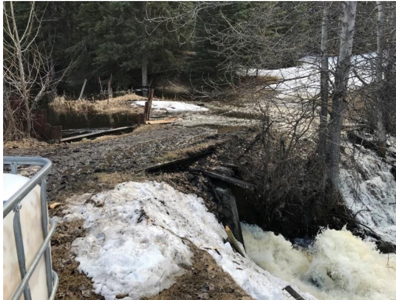
Photo 1: Overtopping and erosion of downstream face of Spokin Lake Dam
