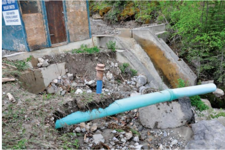
Photo 11: Downstream face of the Cold Spring Creek dam showing path of water to right side of spillway and resulting scour (Credit: Northwest Hydraulics Consultants)
