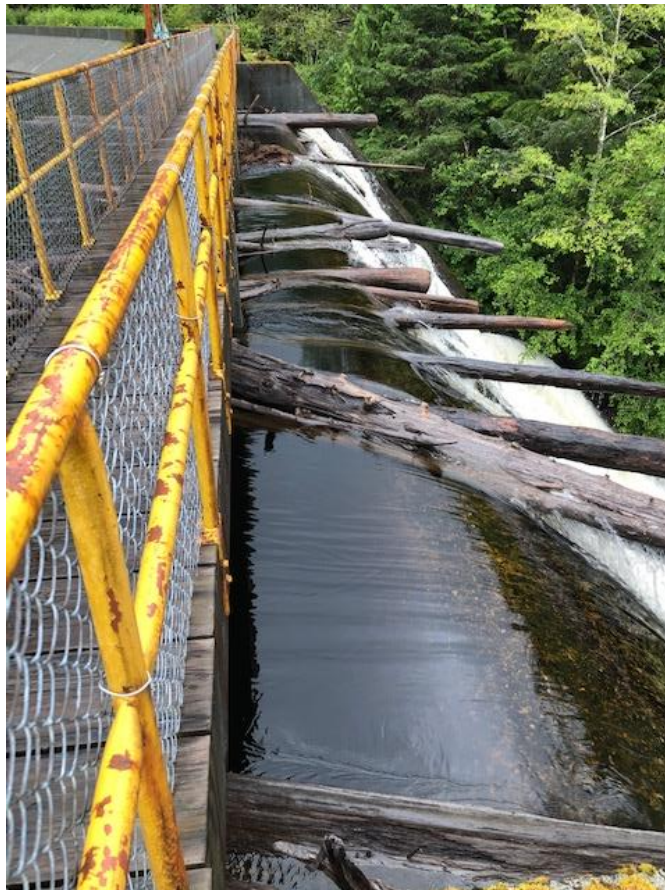
Photo 7: Log debris on the spillway of the Diana Lake Dam
