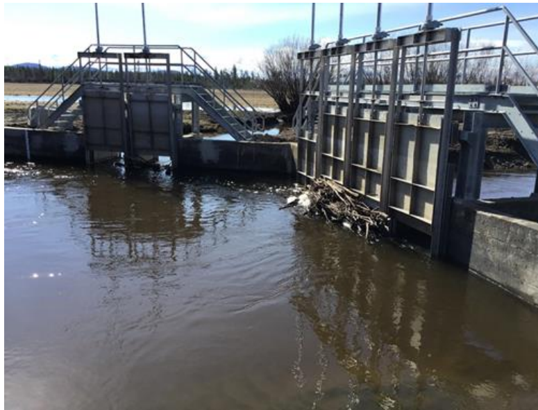
Photo 10: Debris plugging the opening preventing closure of the slide gate of the Anahim Creek Diversion Dam
