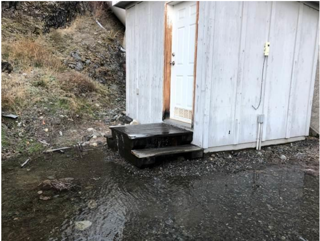
Photo 7: Leakage from the Seton Dam Power Canal weir inside the building
