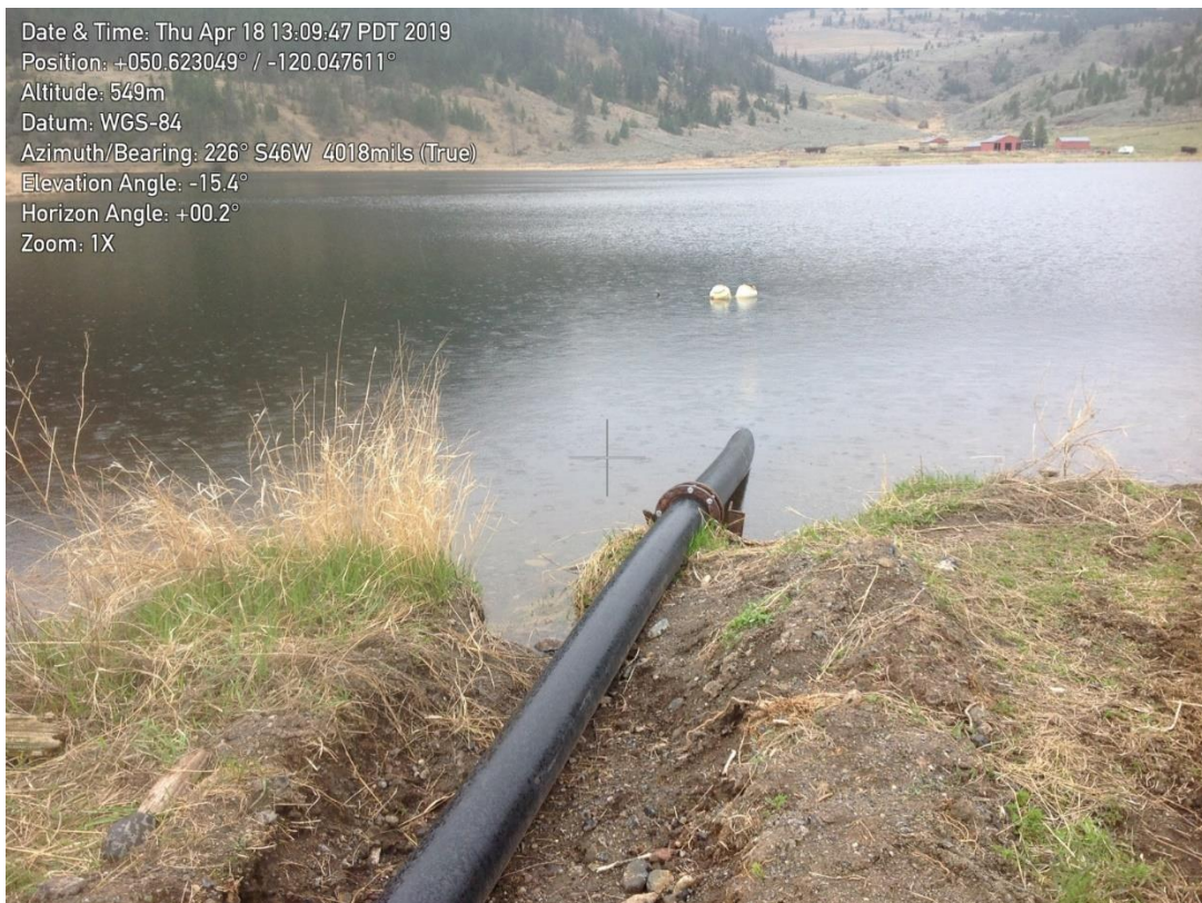
Photo 3: Siphon installed by owner to drain full-supply reservoir of the Upper Buse Lake Dam
