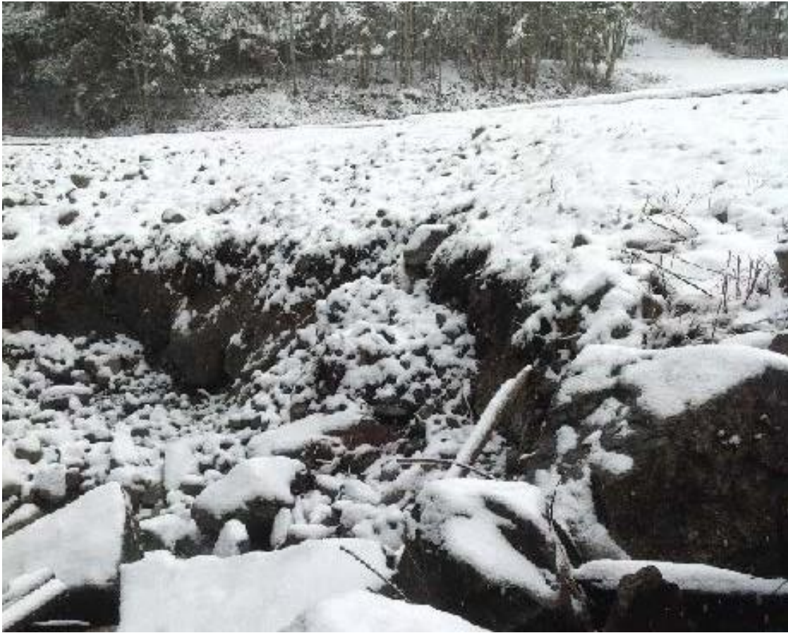
Photo 4: Erosion of the spillway channel of the Cannell Lake Dam
