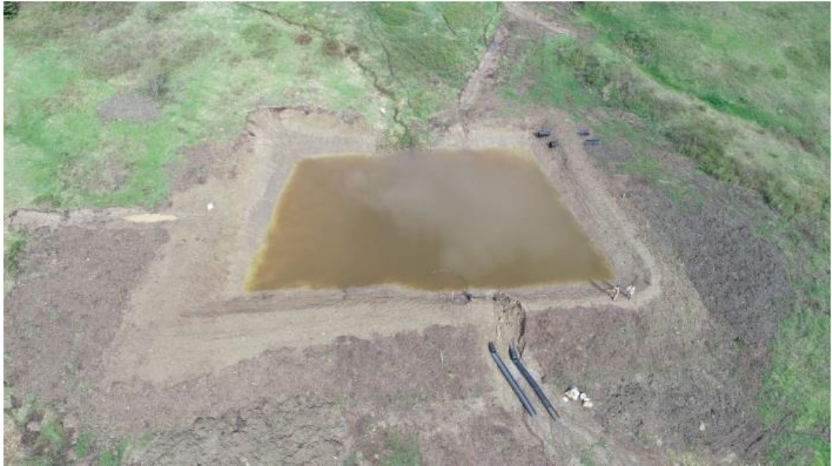
Photo 2: Minor dam failure due to piping around spillway pipe near Hallis Lake Community, Quesnel
