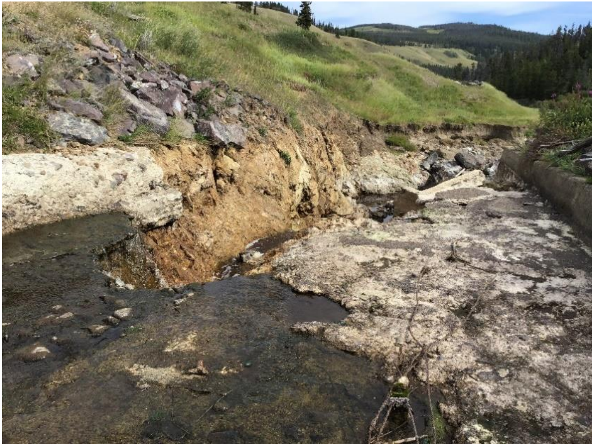
Photo 8: Damage to the spillway bank of the Gaspard Lake dam
