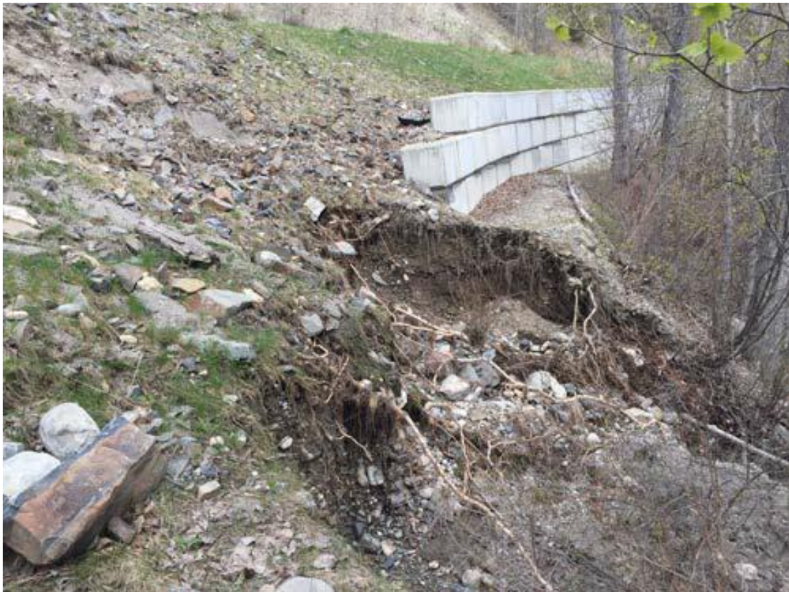
Photo 9: Washout looking upstream towards Aberfeldie Dam
