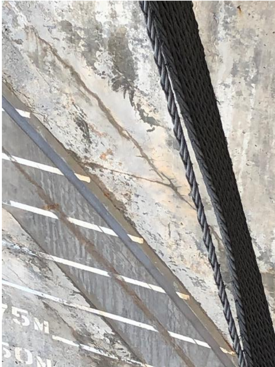
Photo 6: Damaged flat belt used for the actuation of the spillway radial gate with the Skins Lake #2 Dam
