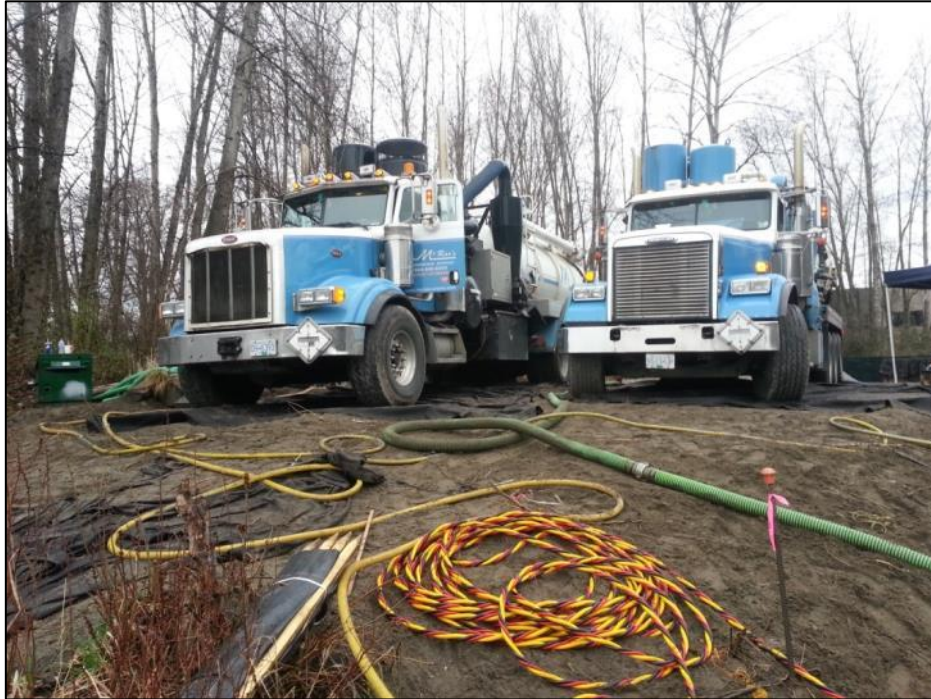
Photograph 21: South facing view of the two vac trucks on the work pads constructed on the turtle beach while recovery was underway
