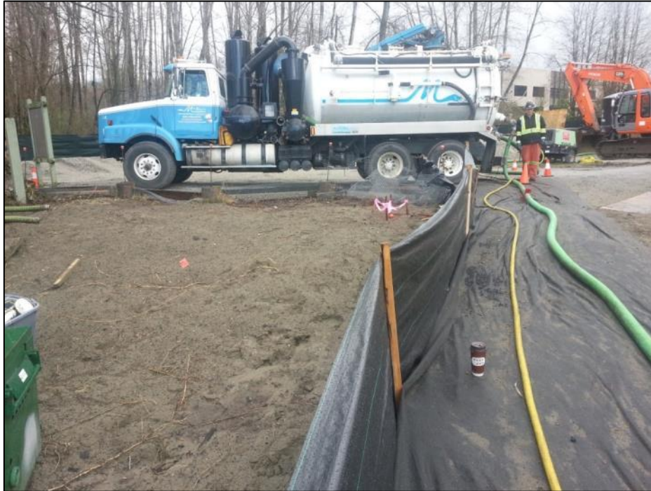
Photograph 19: East facing view of the filter fabric and sediment fence used to protect the turtle nesting beach during coal recovery
