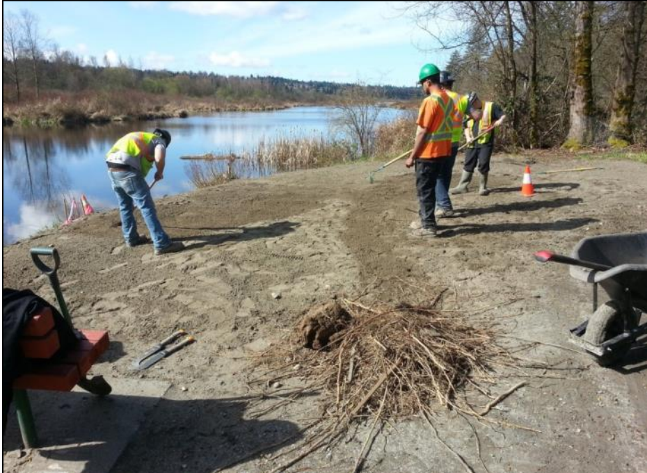
Photograph 25: Crews raking up the turtle nesting beach to reverse any compaction which might have occurred and removing roots and other debris
