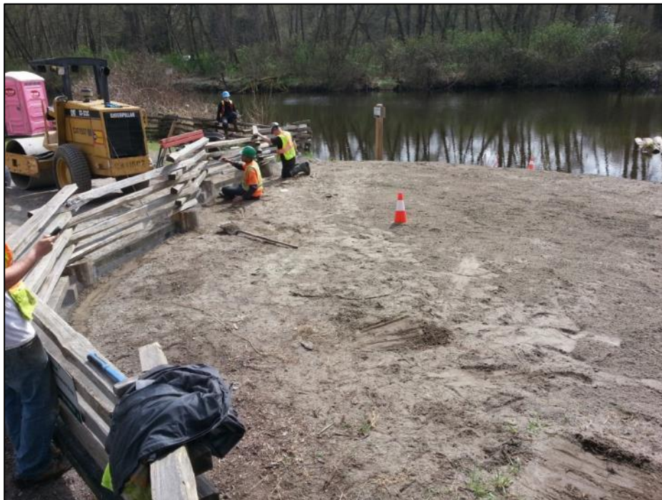
Photograph 30. Southeast facing view of the turtle nesting beach while crews installed the exclusion fence.
