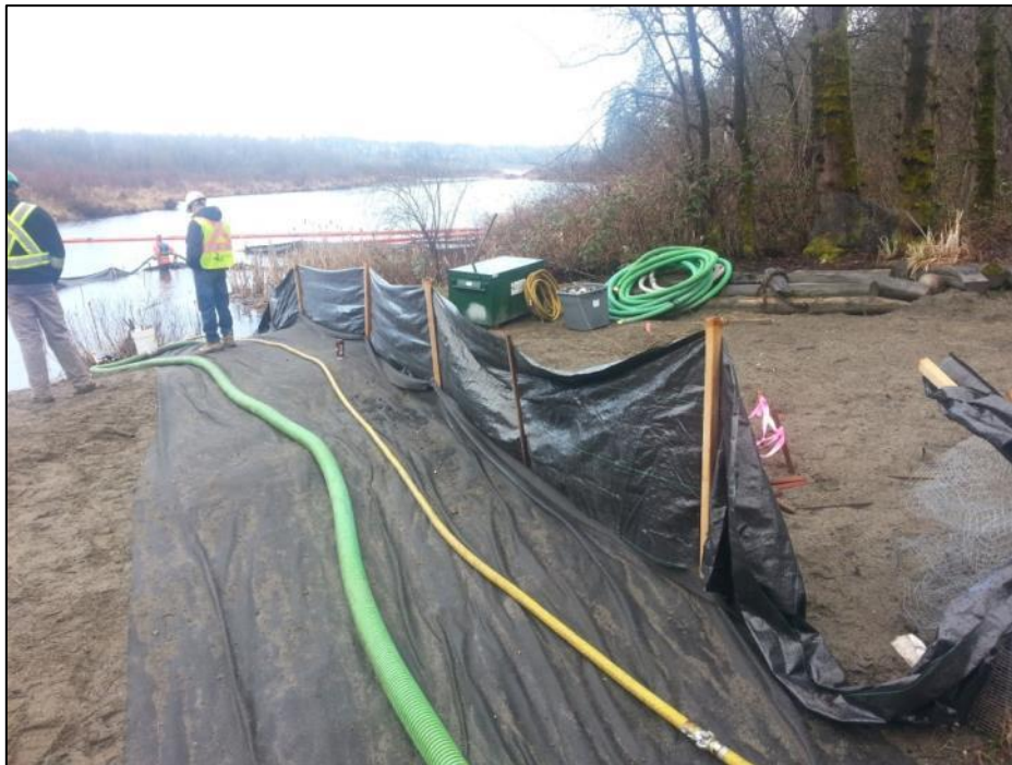
Photograph 20: South west facing view of the filter fabric and sediment fence used to protect the turtle nesting beach during coal recovery
