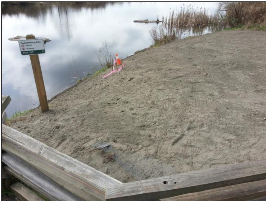
Photograph 28: Southwest facing view of the turtle nesting beach after restoration was complete – fence replaced
