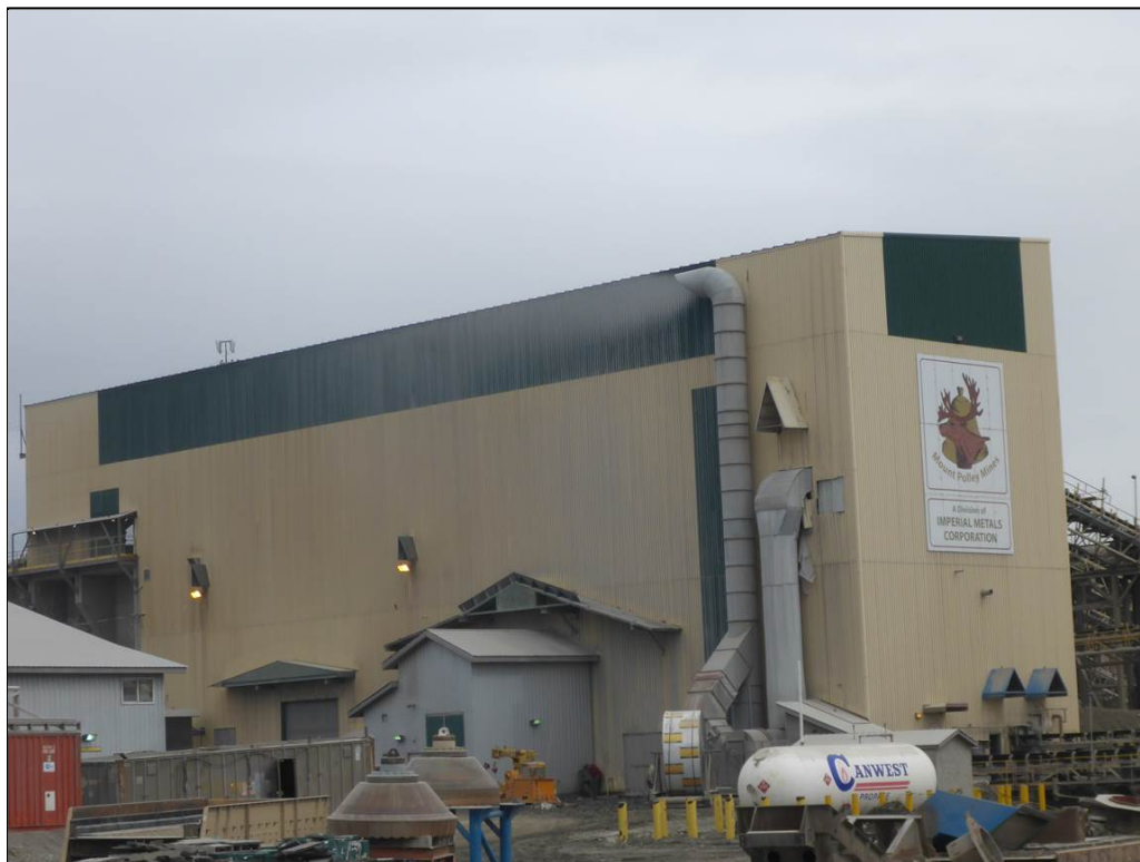
Figure 3. Discharge from the Crusher and Screening Plant. According to staff, in winter the wet scrubber is prone to freezing, resulting in an untreated discharge. Note the staining on the building, caused by the discharge.
