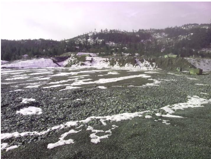
Contact water containment Pond
