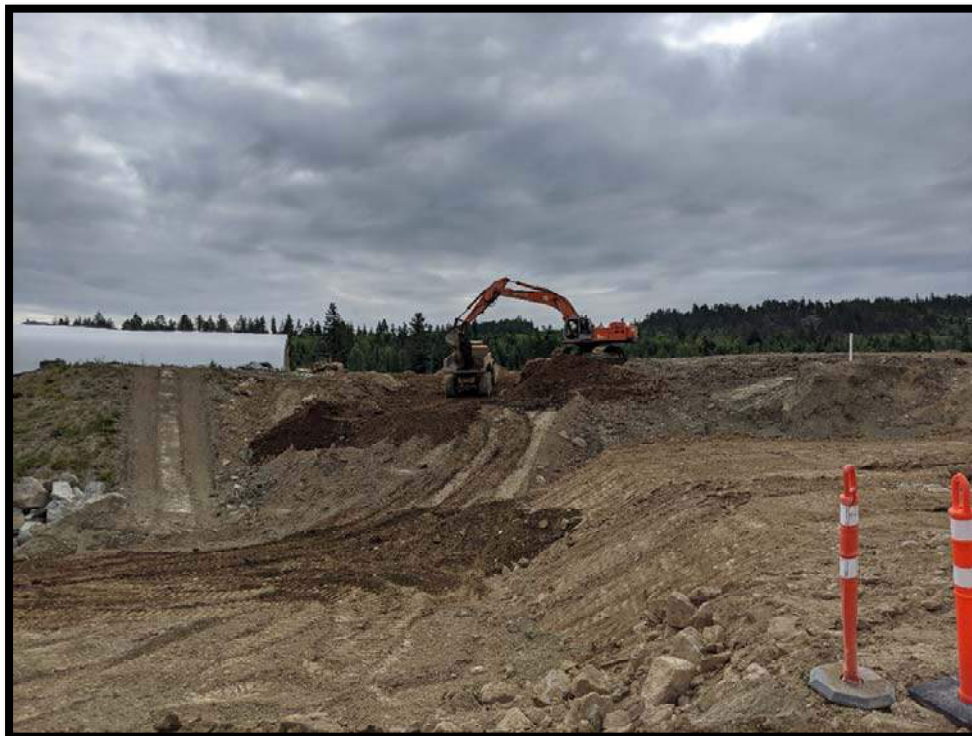
Picture # 2: Looking east towards an excavator loading previously stockpiled material into a rock truck for relocation along the east side of the PEA.
