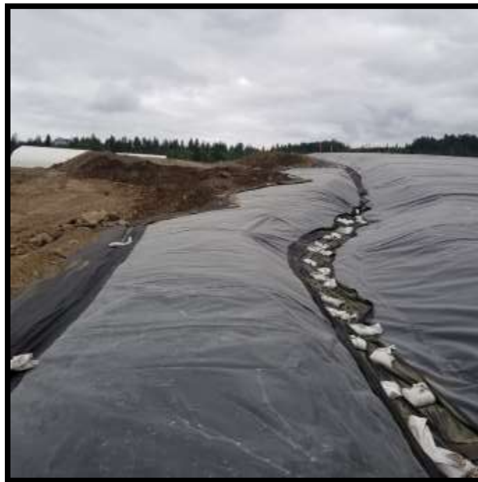
Picture # 4: Soil Placement via Staggered Completion on the North Face – Looking East
