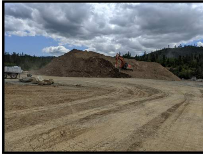
Picture # 1: Contractor stockpiling soils from 2251 Bear Mountain Parkway to the south of the PEA.
