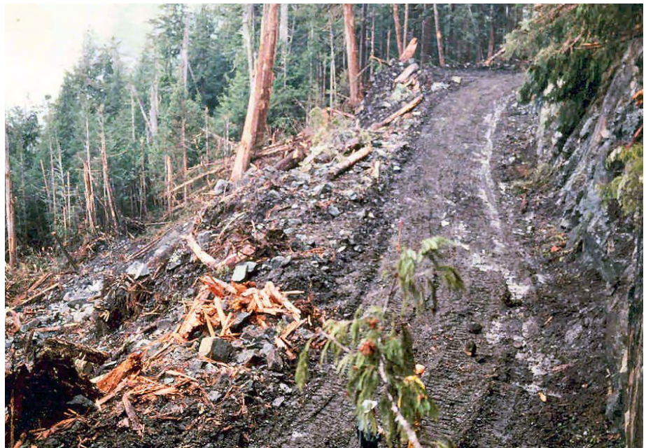
FIGURE 5 Failure of an organic soil loaded with sidecast material, Security Bay (Photo: Jim Schwab).
