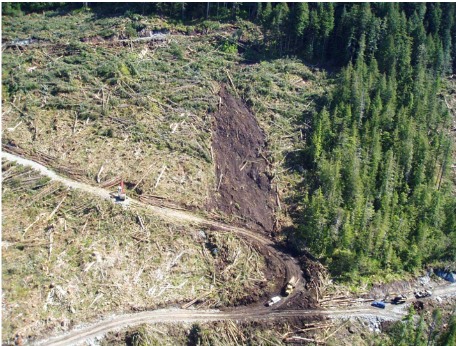
FIGURE 6 Landslide triggered in shallow organic soil during road construction, Kennedy Island. Landslide debris struck a crew truck parked on the switchback. Timber felling occurred post-landslide (Photo: Jim Schwab).
