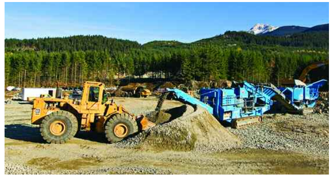
Previous page and above: Construction is underway at the site of the Olympic and Paralympic Athlete's Village (also called the Legacy Neighbourhood) in Whistler. Photos by David McColm.
