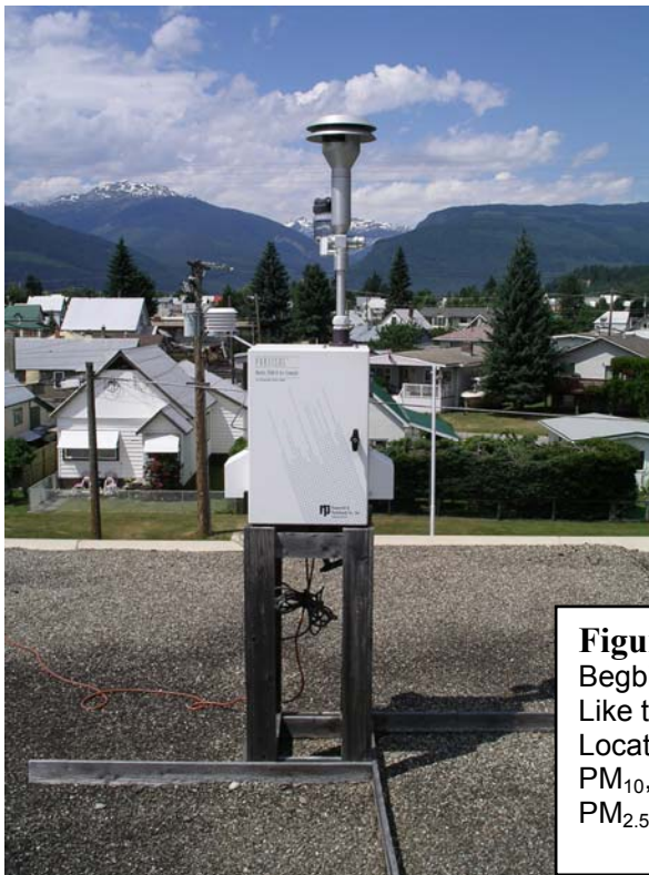
Figure 3. Periodic maintenance is performed on the high-volume (Hi-Vol) manual sampler on the roof of the Fire Hall. It collected a sample over a 24-hour period every sixth day, until July, 2007
