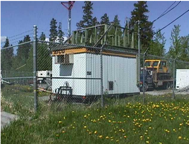
CBC Transmitter site looking towards the west
