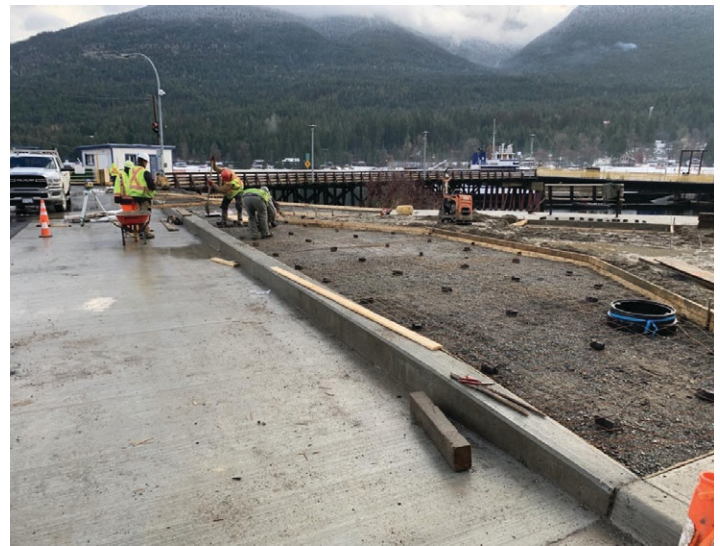
Building out the form for the bus pad landing at Balfour terminal.
