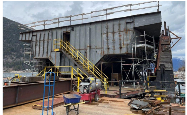
The bulk of the vessel hull assembled on the floating dry dock.
