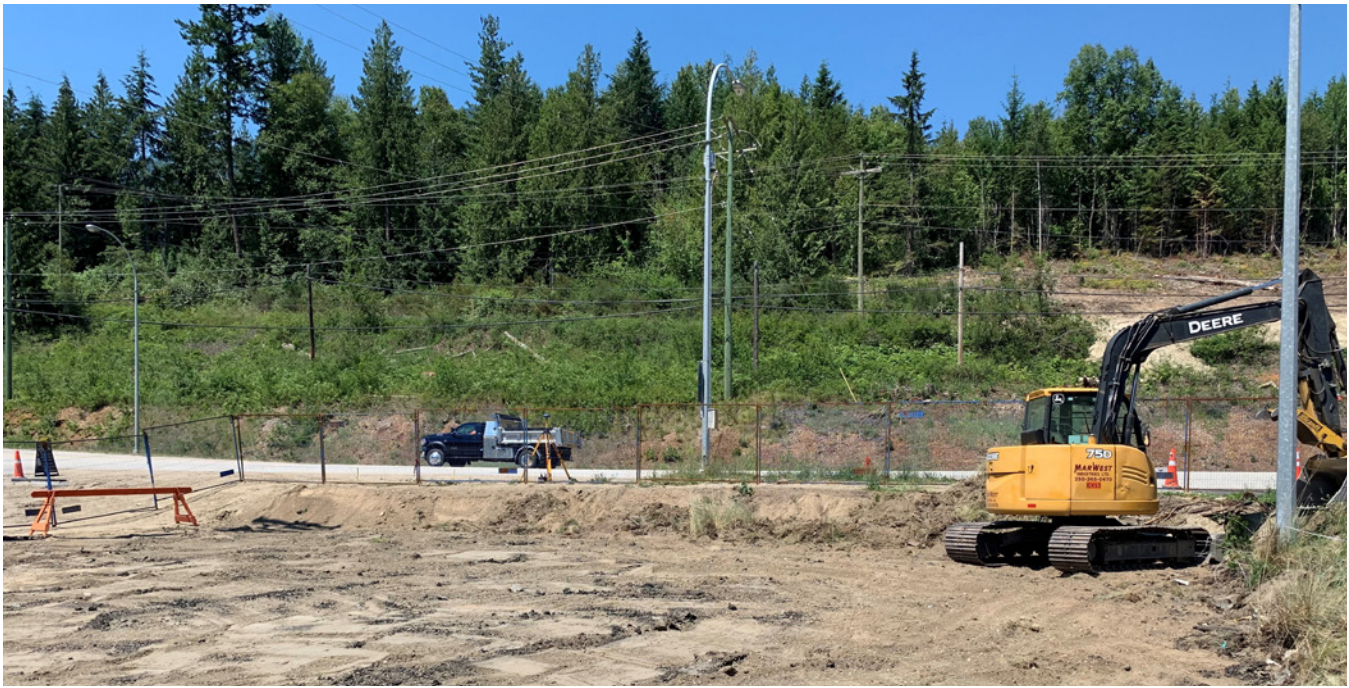
Excavation for the new washroom building in the Balfour terminal currently underway.
