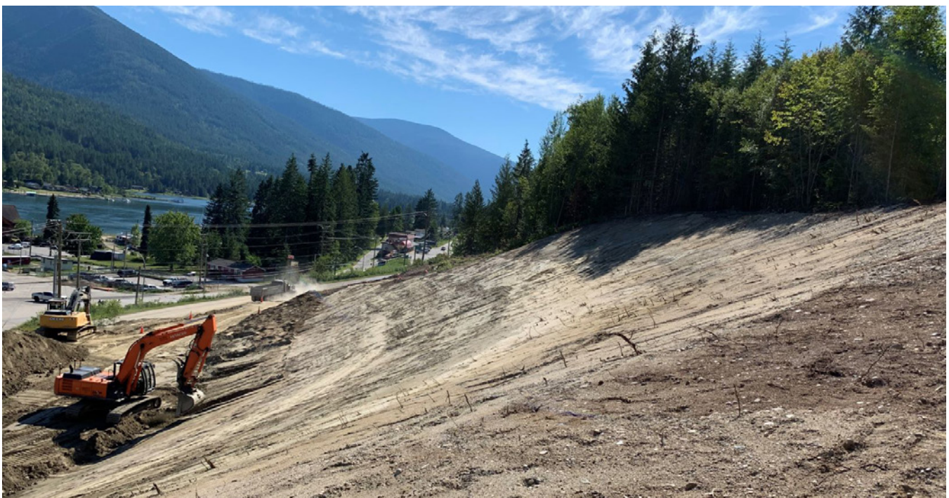
Grading of the steep slopes along Highway 3A are currently underway to support the realignment of the Upper Balfour Road and Busk Road intersection.
