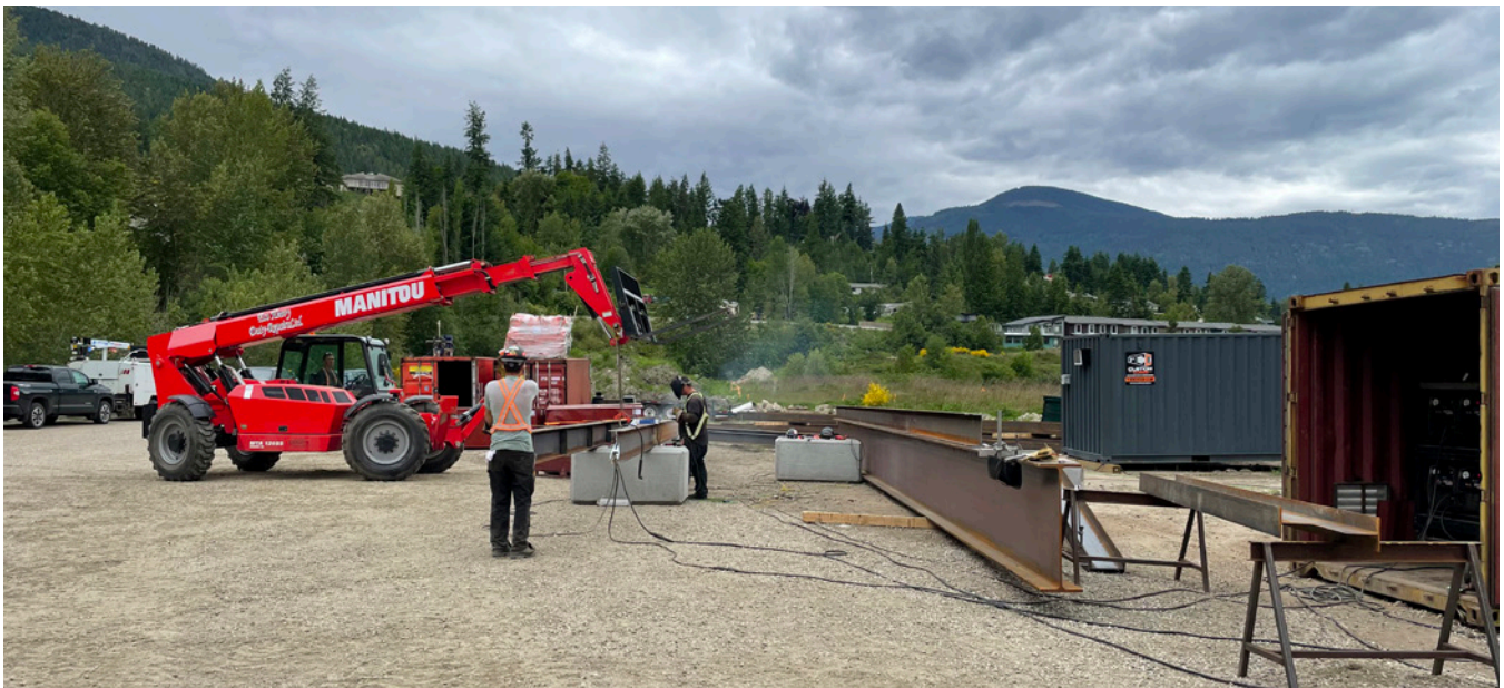
Crews are safely progressing the infrastructure needed to receive the first modules of the new vessel later this summer.
