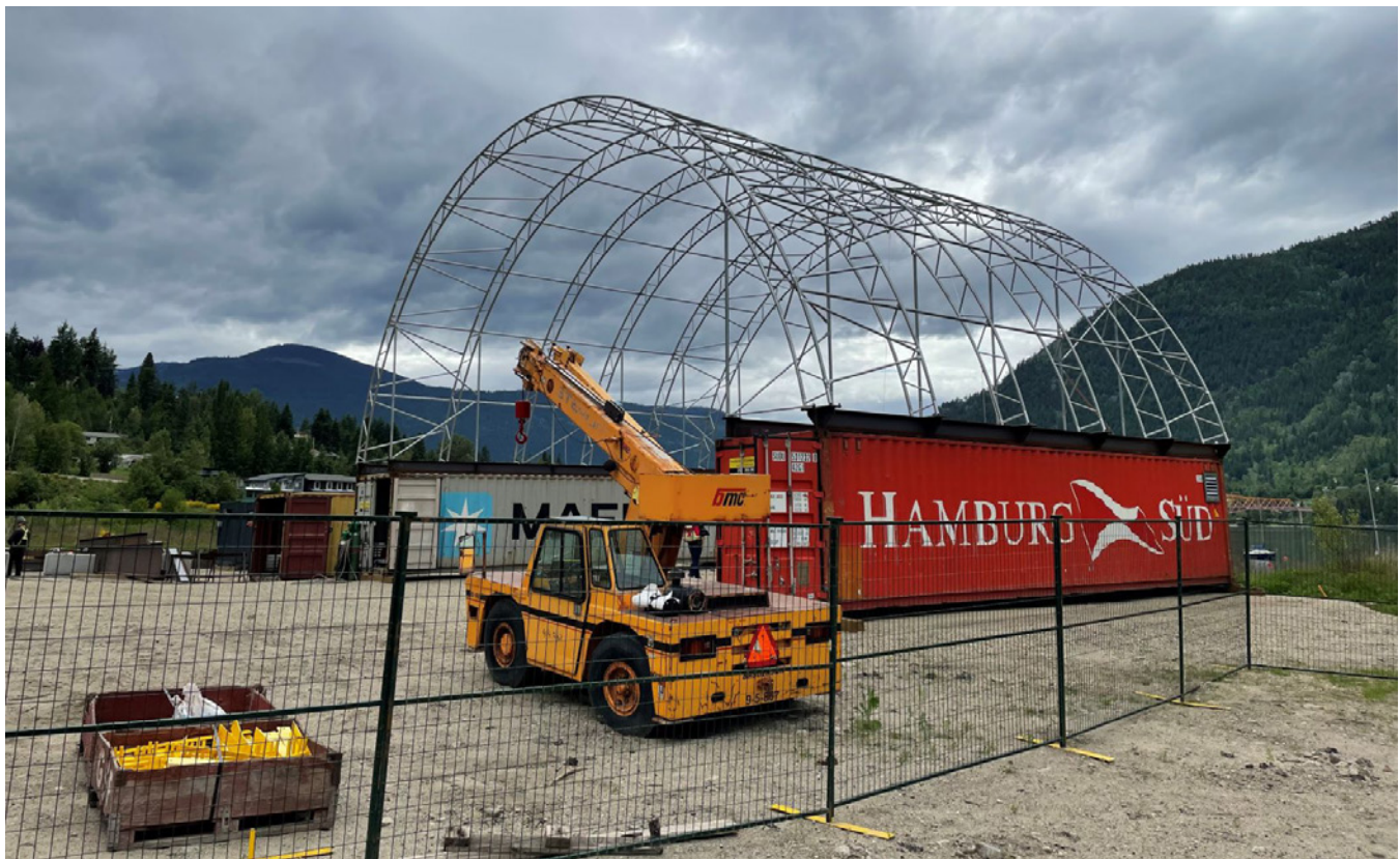
Site preparation activities, such as the building of this shelter, are underway at the assembly yard in Nelson, B.C.
