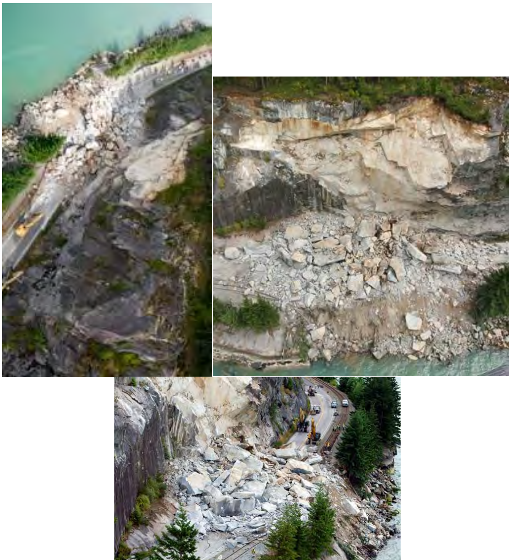
Rock Slide - Highway #99 Porteau Cove
