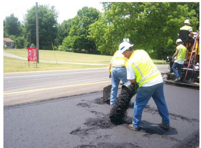
B6 - Filling the hole left behind by vertically dumping new asphalt mix.
