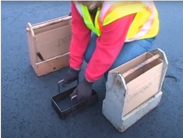
C3 - Placing sampling template at selected location on newly placed asphalt mat.
