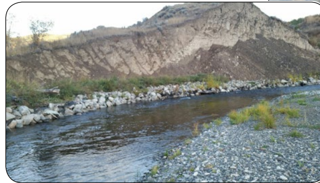
▲ After: Rock and wood structures were installed, and vegetation planted, to reduce the cutbank's erosion and the flow of sediment into the river.
