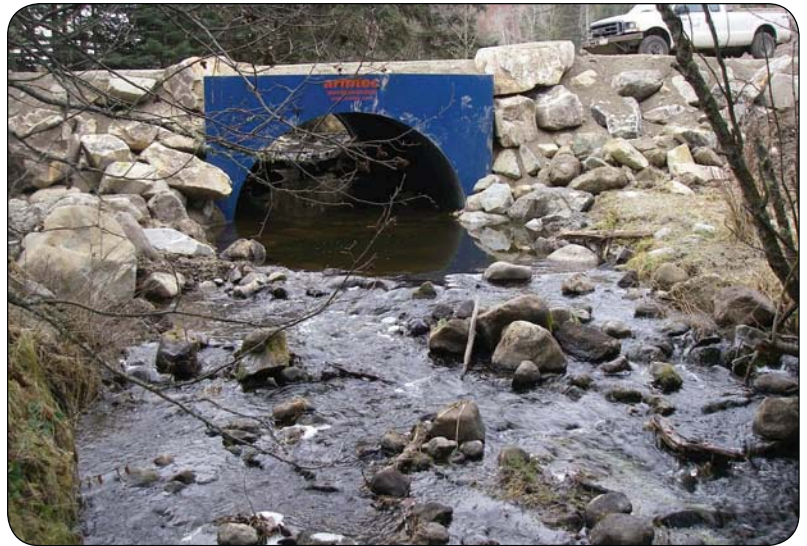
After: The new culvert maintains biodiversity by improving access to fish habitat.
