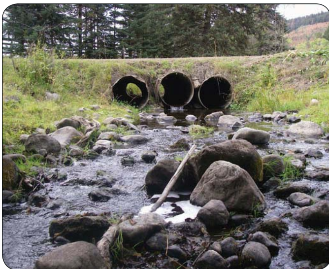
Before: The culvert at St. Laurent Creek limited the passage of fish.
