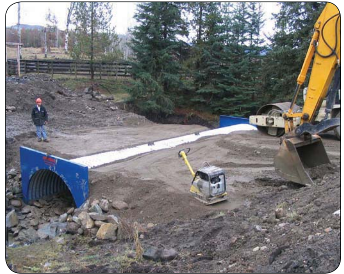
Construction at St. Laurent Creek, south of Chase, funded by the Culvert Retrofit Program.
