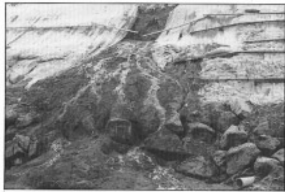
Fig. 18 High seepage flows from a slope.
