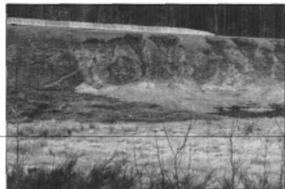
Fig. 13. Surface slumping on a fill slope in till.
