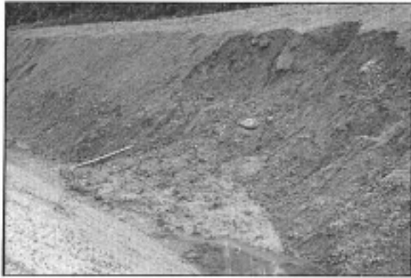
Fig. 19 Surface slump in relatively low slope.
