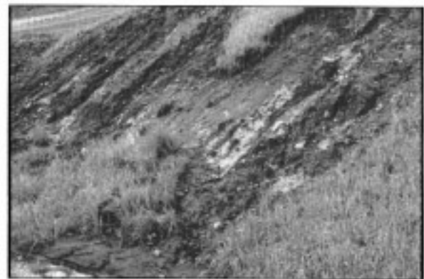
Fig. 14. Failure of topsoil placed on a smooth, 1.5:1 slope.
