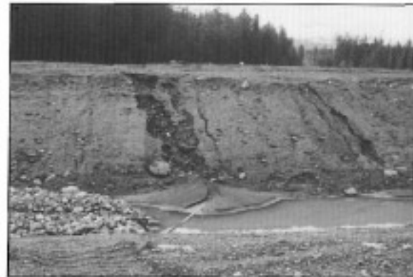
Fig. 5 Severe gullying from concentrated surface flow at the top of a cut slope.
