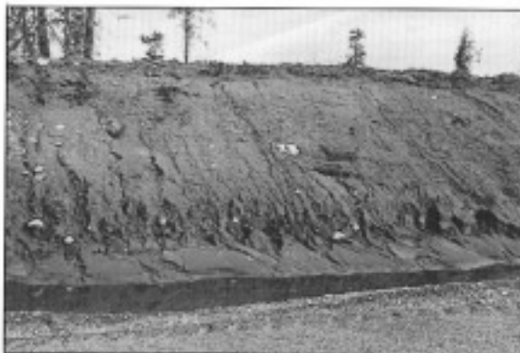
Fig. 2 Example of rill erosion
