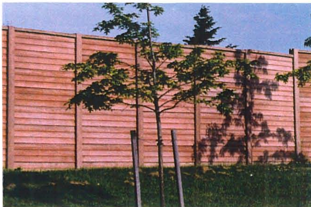
Figure 2.3; A 3 m High Precast Concrete Noise Wall at the McKenzie Interchange Near Victoria
