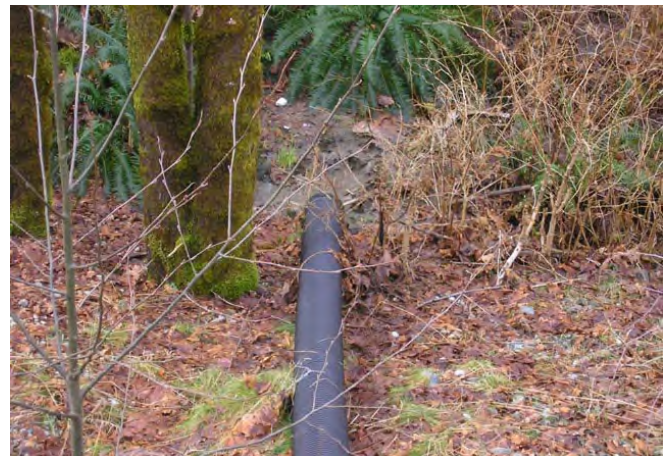
Photo 4. Drainage collected along asphalt curb discharges through downspout pipe away from sensitive watercourse. Outlet is armoured with rock splashpad to prevent erosion.
