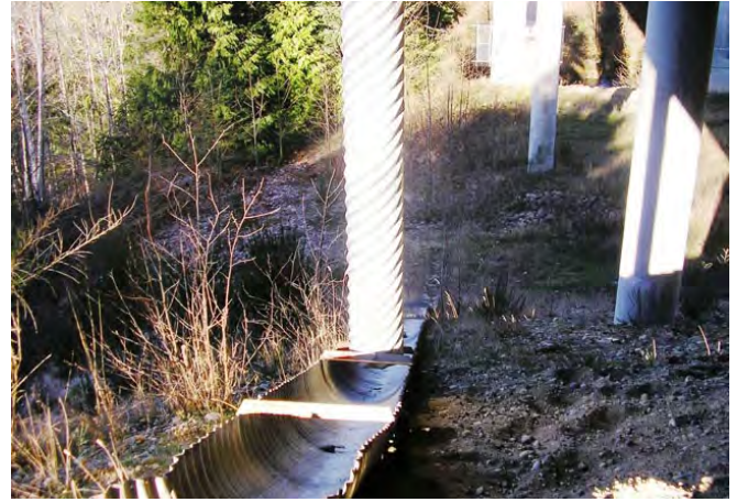
Photo 8. Vertical collection culvert discharges to flume and then rock splashpad to avoid bridge endfill saturation and erosion.
