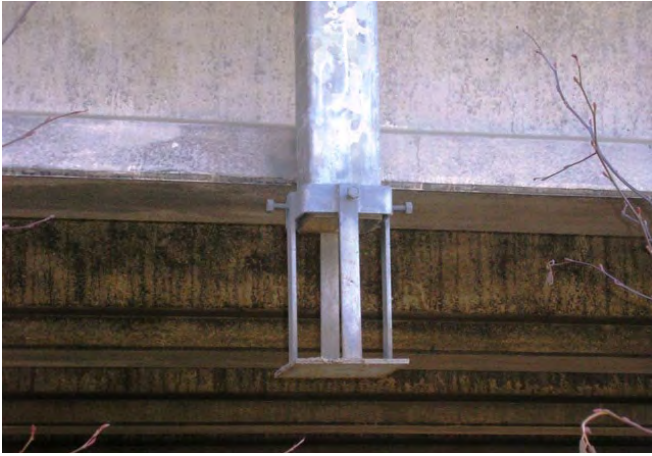
Photo 7. Spray dissipater at end of downspout dissipates discharge to avoid erosion and fill saturation.
