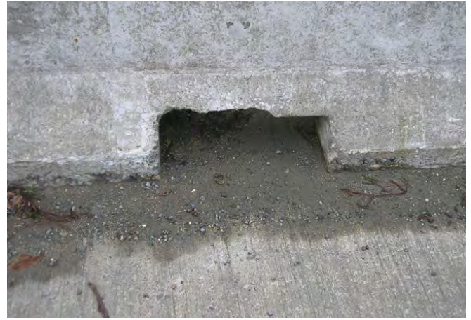
Photo 2. Bridge parapet scupper opening to collection trough requires periodic cleanout because of susceptibility to debris plugging.
