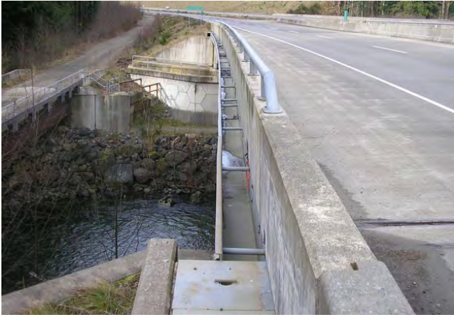
Photo 1. Drainage collection trough on outside of bridge parapets. Metal plates in foreground cover cleanout catch basins.
