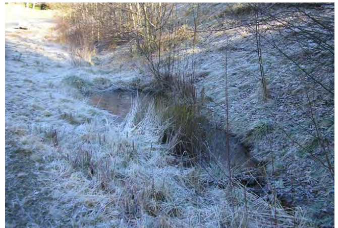
Photo 6. Vegetated ditchlines with constructed ditchblocks create settling cells that treat and filter road runoff prior to it reaching a watercourse.
