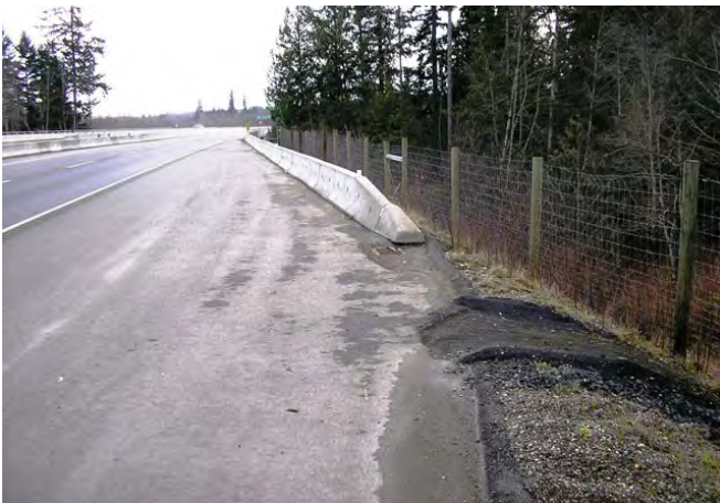
Photo 3. Asphalt curb at bridge approach intercepts grade runoff prior to bridge deck and directs it through asphalt spillway to prevent embankment erosion and downstream sedimentation. Grated catch basin at end of concrete barrier also collects runoff prior to it reaching the bridge deck and sensitive watercourse.
