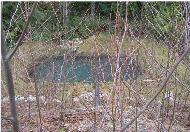
Photo 5. Highway drainage collection pipe discharging to constructed settling pond enables sediment settling.
