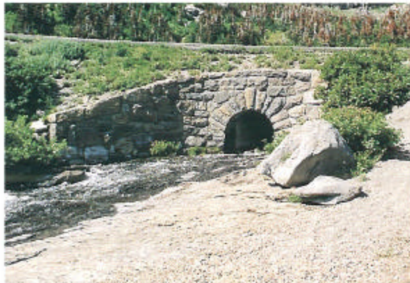
Figure H-11 A well designed culvert headwall - appropriate to a highly visible parkway site.
