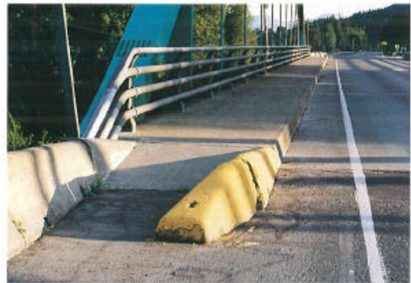
Figure H-27 Avoid the use of paint on concrete traffic barriers
