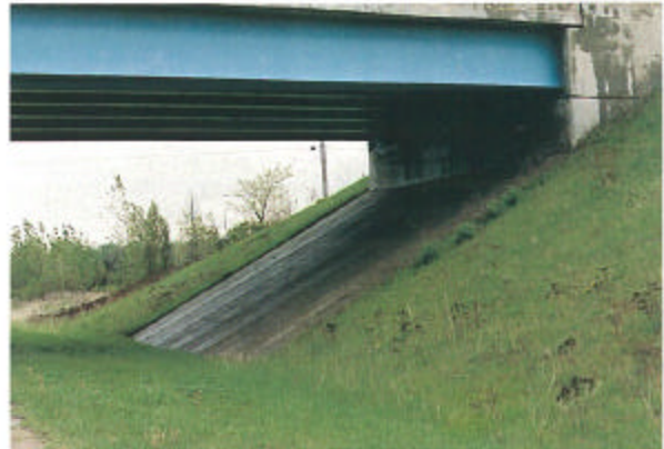
Figure H-20 Example of a rural bridge slope finished to allow ease of maintenance.
