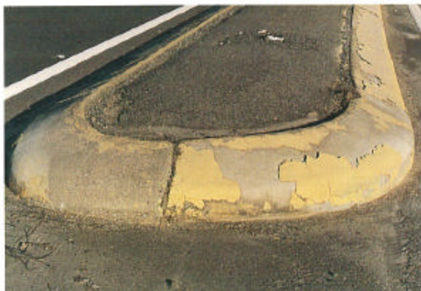
Figure H-37 Minimize the use of paint on curbs, or develop higher maintenance standards to minimize peeling, cracking condition.
