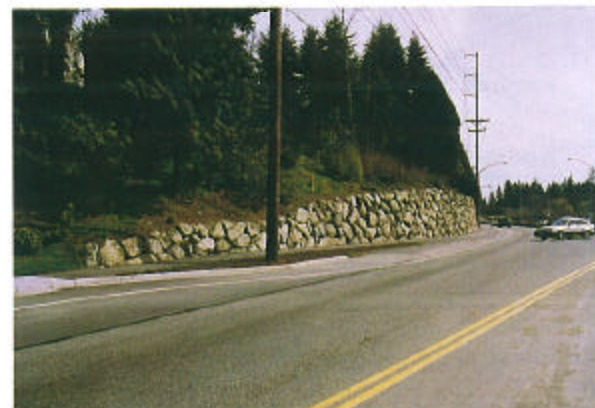
Figure H-25 An example of a retaining structure using locally available materials.
