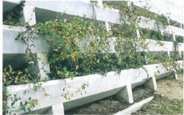
Figure H-12 This retaining structure is well textured with linear planting strips and vegetation. This scale of detail is appropriate when viewed at highway speeds.
