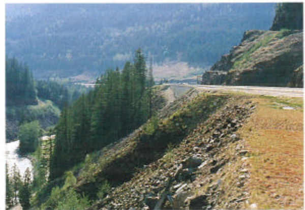
Figure H-4 The wall in the background allows the vegetation downslope to be retained. The foreground shows the impact without the wall.
