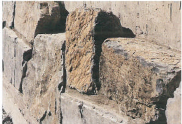
Figure H-13 Stone veneer in process. This would be appropriate on a Parkway project, or area of close public inspection.
