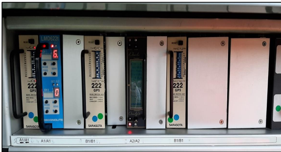
Figure 9. Cabinet Blanking Plates
