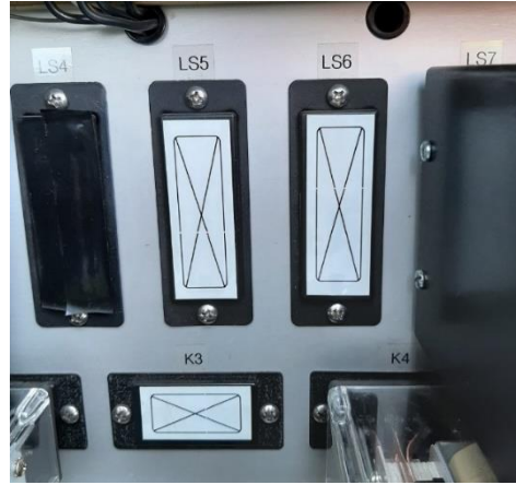
Figure 22. TS1 Typical Unused Load Switches and Flasher Socket Label
