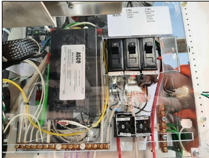
Figure 10. 'P6' Cabinet Power distribution
