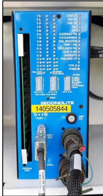
Figure 16. Malfunction Monitor Unit (MMU)
