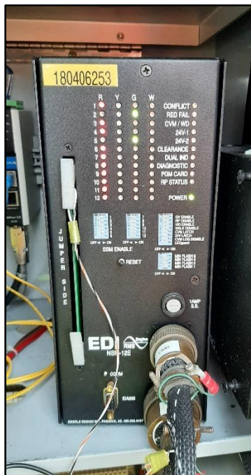
Figure 8. 'M' Cabinet Conflict monitor unit.
