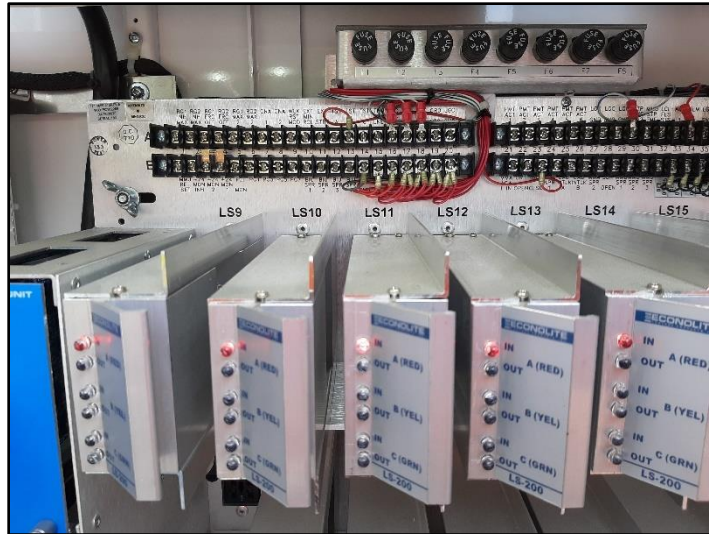
Figure 13. 'P6' Load Switches
