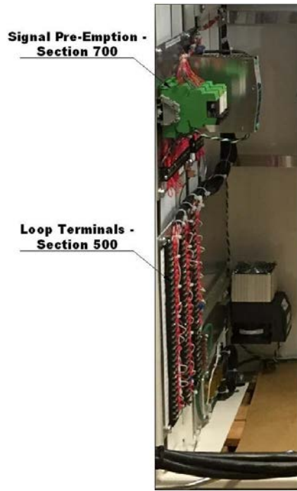
Figure 21. The P6 TS2 Traffic Controller Left Wall Equipment
