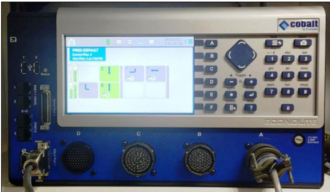
Figure 23. The Econolite Cobalt Type 2 Controller Unit
