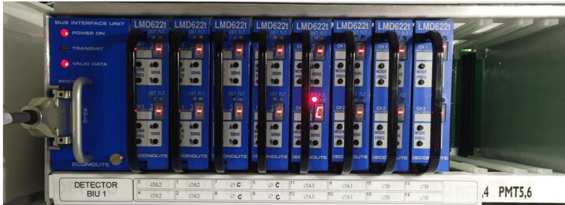
Figure 29. TS2 Detector Rack
