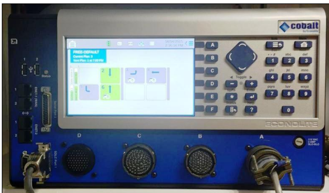
Figure 2. The Econolite Cobalt Type 2 Controller Unit
