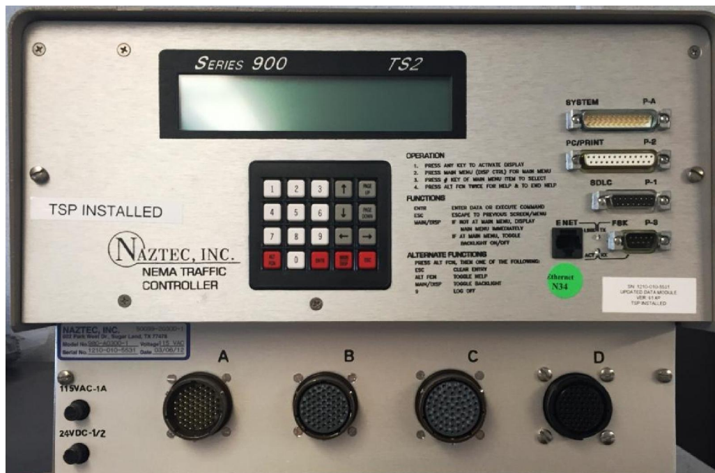
Figure 3. The Trafficware/Naztec 980 Type 2 Controller Unit
