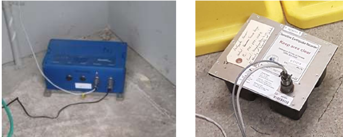
Figure 3.1 Typical BCSIMS Earthquake Sensors on foundation.
