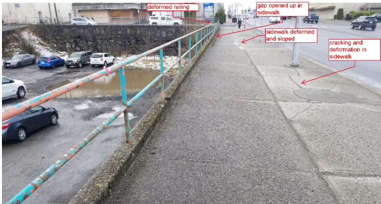
Figure 2: View of sidewalk above rock wall along 2 Ave W. Cracking and sidewalk deformation visible. Looking south from bus stop.
