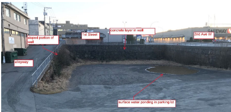
Figure 3: View of rock wall looking southwest from the NE corner of the parking lot.
