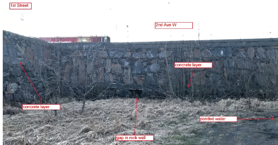
Figure 5: View of rock wall at the corner of 1st Street and 2nd Ave with vegetation and gap visible in the base of the wall. Taken from the south end of the parking lot looking west.
